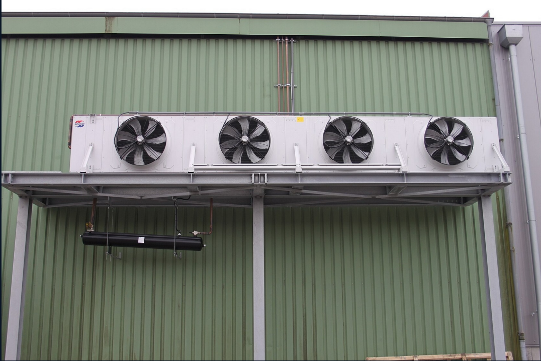
Air-cooled condenser with four fans, on the wall of a cold store
